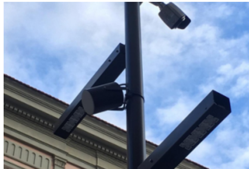
Smart CCTV Security
